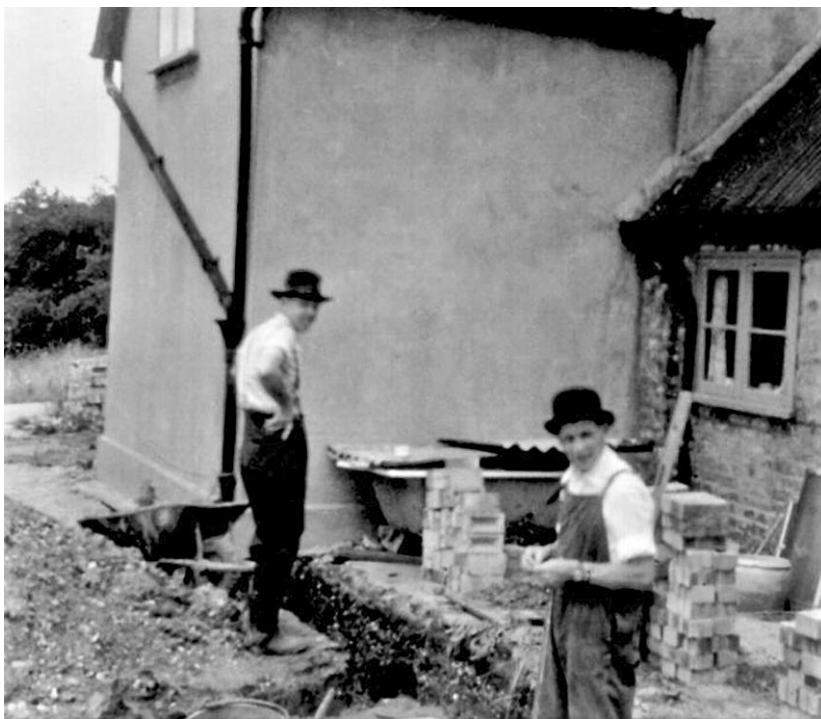
Image 15. Work begins on construction of the extension at the rear of the lodge in 1961.
